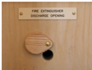
Proper fire port into the engine space from the cabin.
