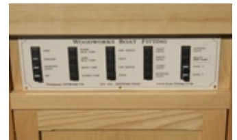
Logical electric panel with circuit breakers.
