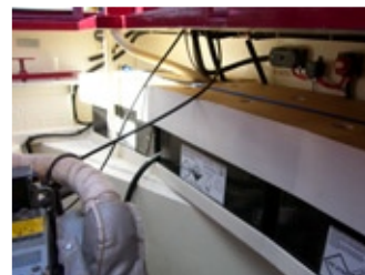
Massive domestic battery bank securely restrained and covered.
