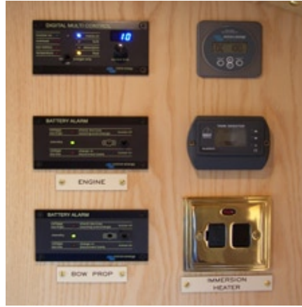
Battery system and tank monitors are positioned on the galley bulkhead.
